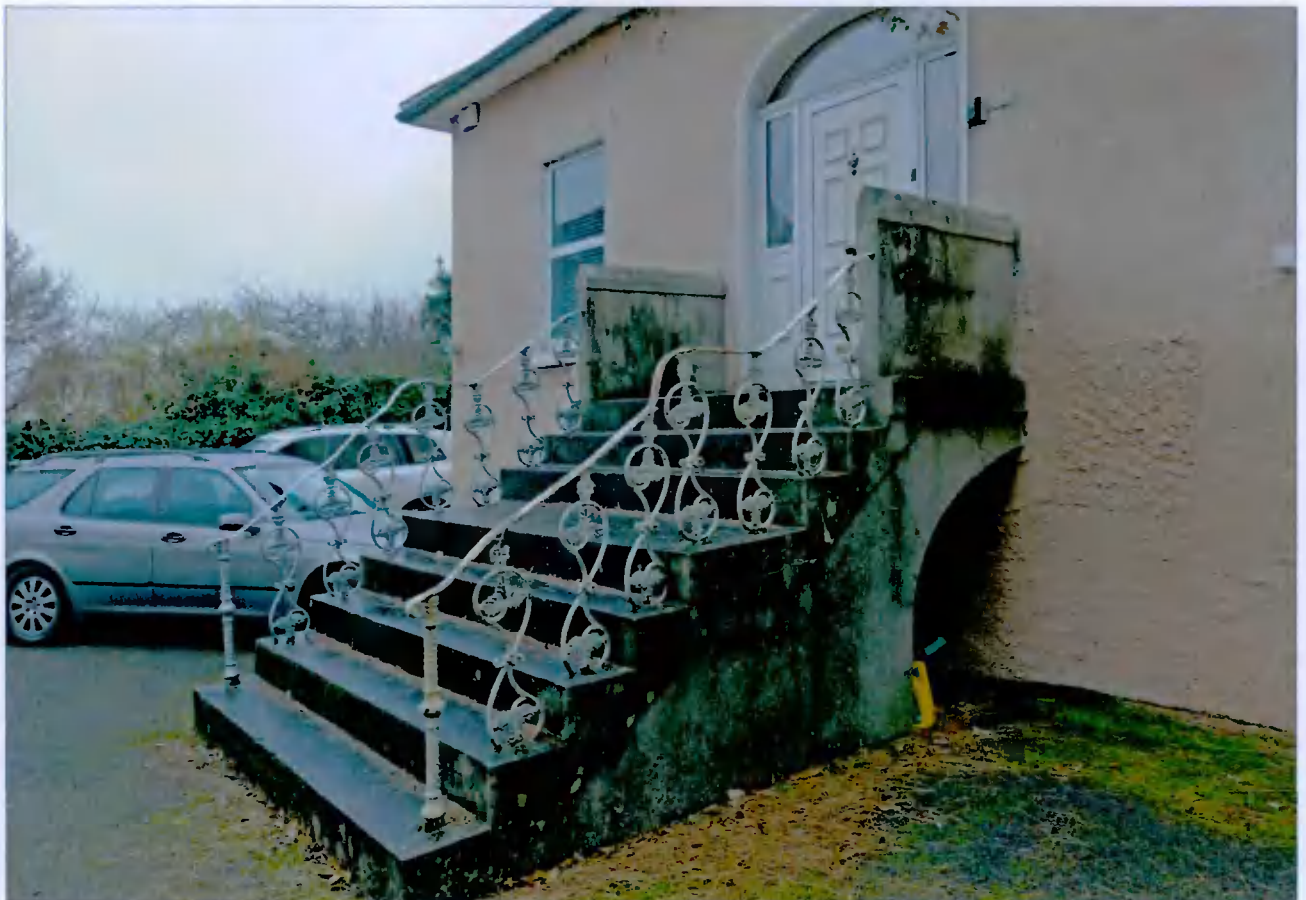
Front Steps. It is proposed to overhaul and repair the front steps where required.
