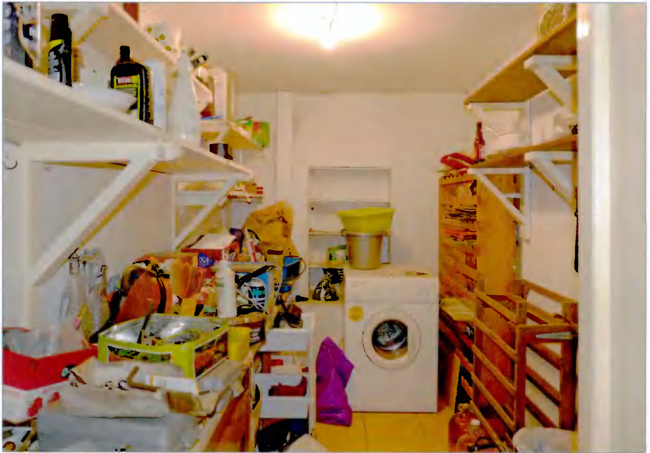
Central room at the west end of the lower level - ie: below the entrance hall. It proposed to convert this room into a bathroom.
