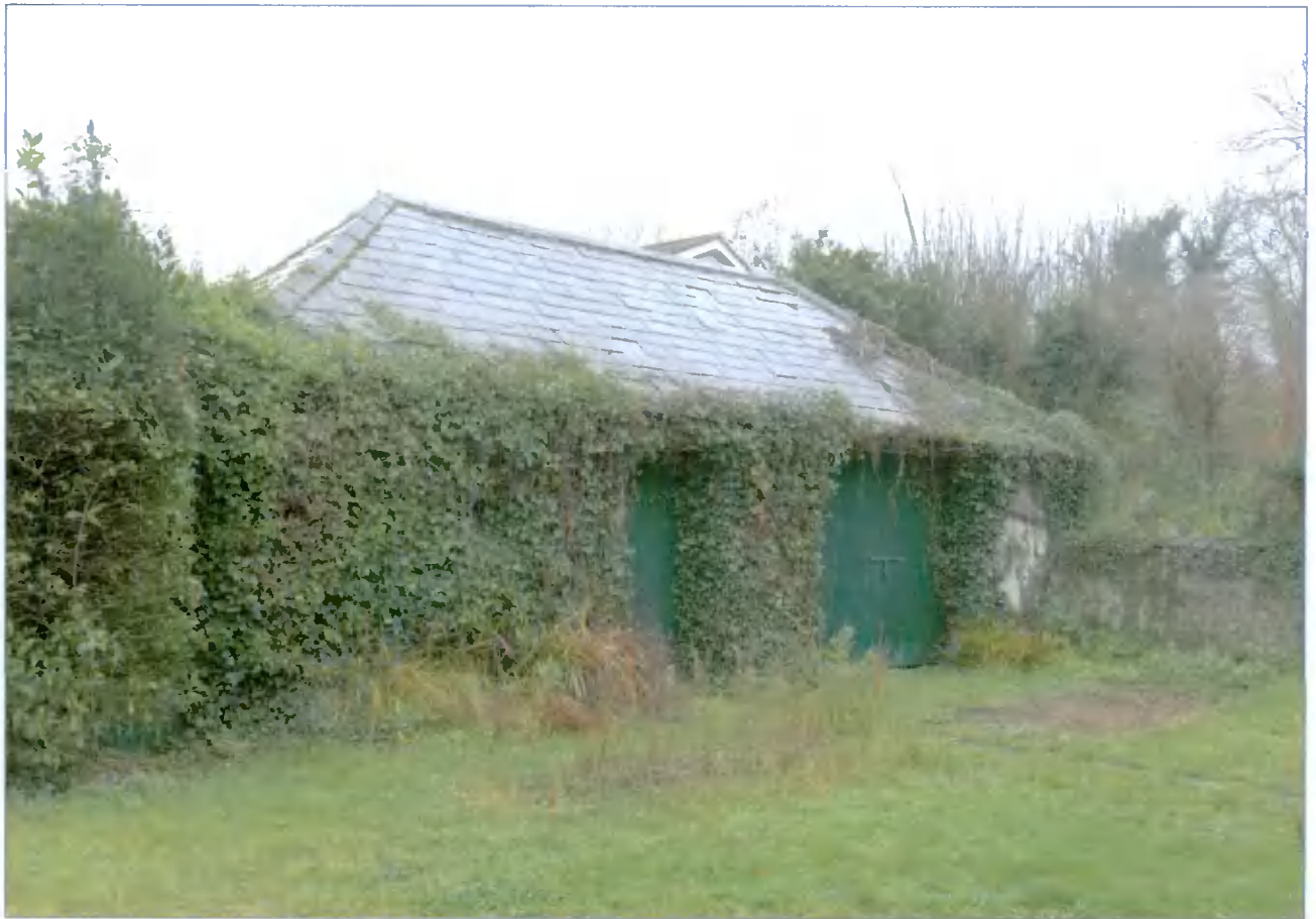
South west outbuilding. It is proposed to overhaul and repair this outbuilding.
