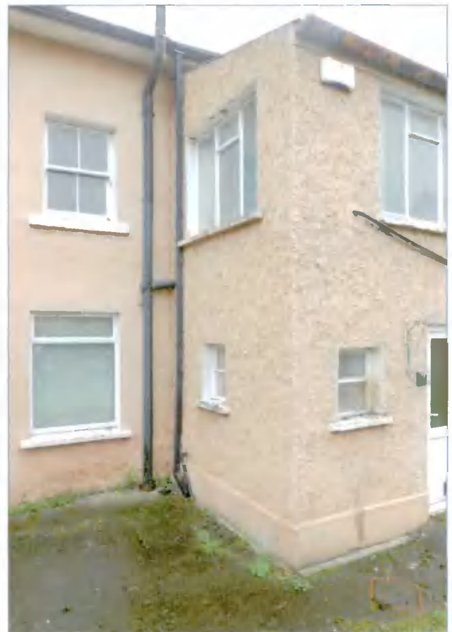
South east corner. A new return is proposed extending across the rear of the house incorporating part of the old.
