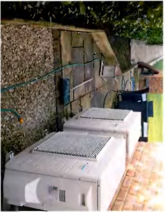
Top: Solar Panels Bottom: ASHP
