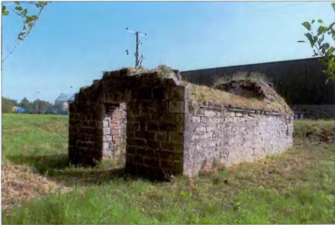
Plate 1: North-west entrance elevation of former gun powder store with south-west side elevation. Gravel surface to approximately 1.5m perimeter of structure. Annual light vegetative growth is trimmed back twice per year in accordance with conservation recommendations by site maintenance staff.
