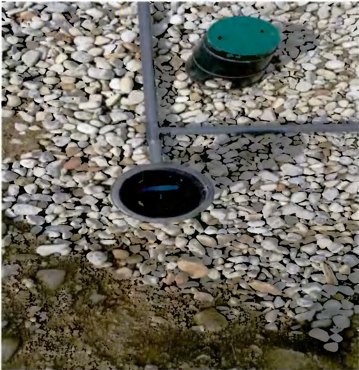
Photo 4 - Flush Valve Taps
