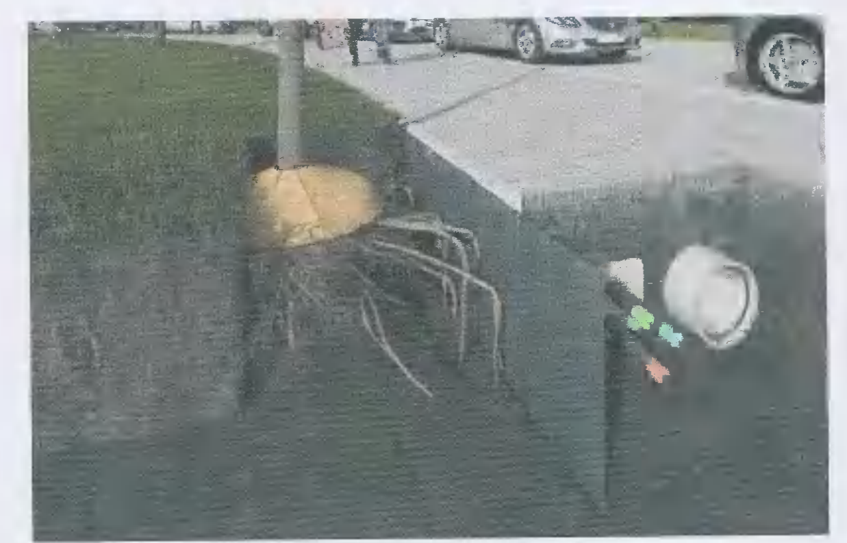
Root barrier to ensure a separation between the tree root system and the installed services
