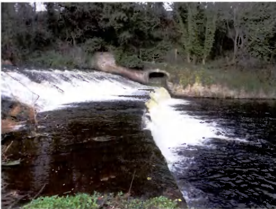
Plate 3.15 The River Dodder at Dodder Road showing one of many major weirs along the middle and lower reaches of the river
