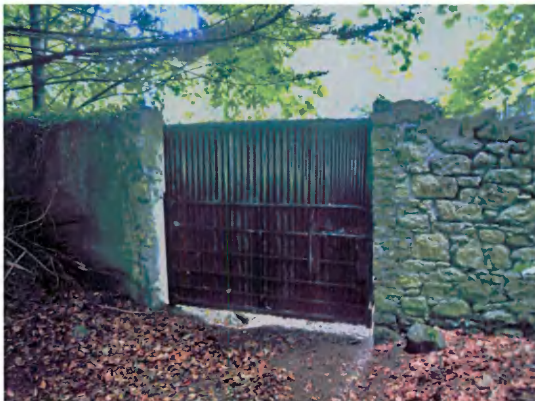
16 Gate in stone wall running east -west across site, seen from south
