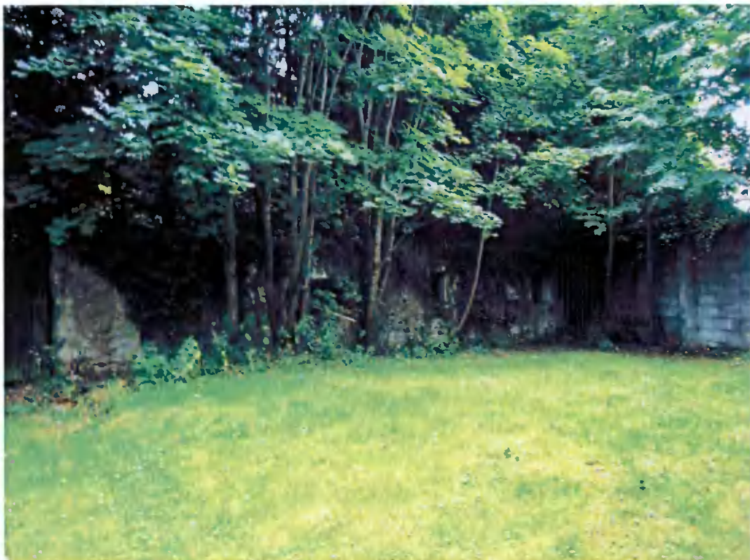
18 Western end of on-site stone wall from north joins boundary wall at Grangebrook Avenue
