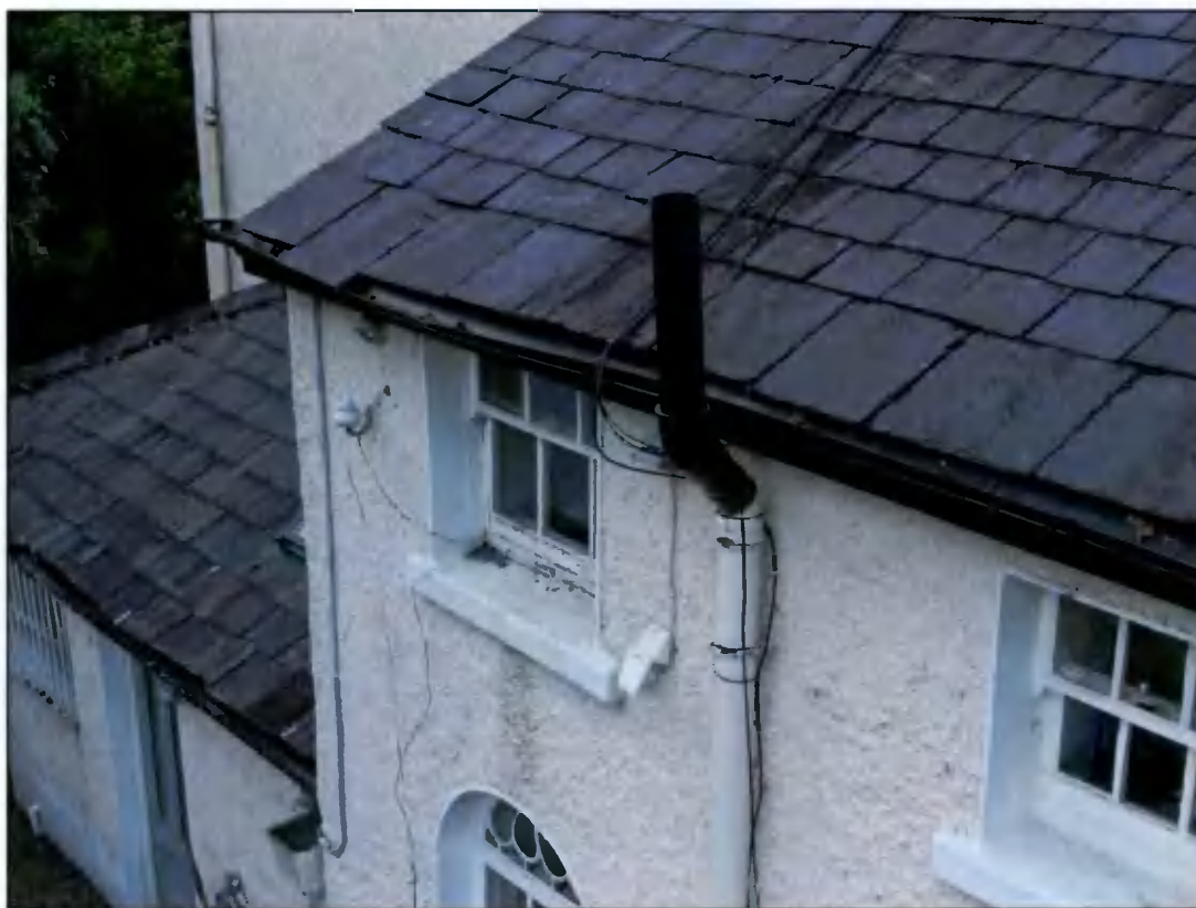
Figure 37: Areas of roof where slate has become detached
