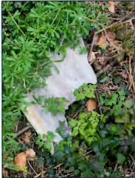
Figure 24: Fragment of old roof covering of shed that may contain asbestos
