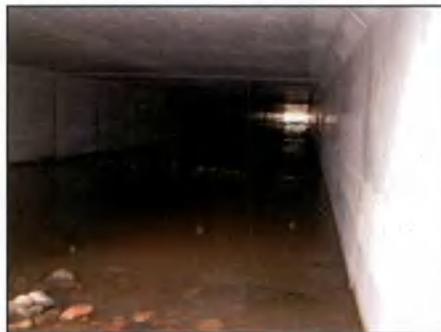
Excessively long culvert resulting in habitat loss and reduced productivity due to inadequate light penetration.
