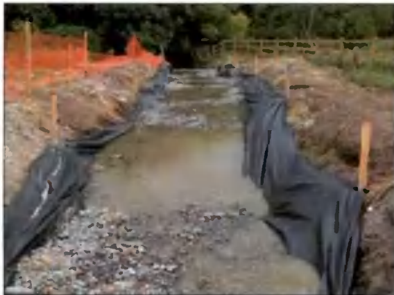
Terram lined (to prevent erosion) silt control pond outlet channel showing gravel acting as filter medium for silt removal.
