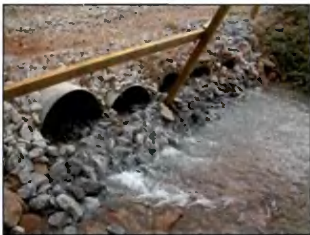
Temporary crossing impassable to fish life.
