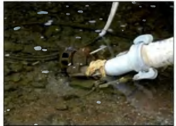
Continuous abstraction using submersible pump. No screening in place to prevent the entry of e.g. juvenile fish species to the pump. Unacceptable practice.
