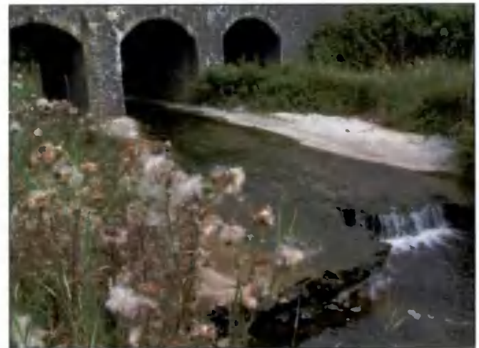
Apron/scour slab inaccessible on its downstream end to fish life because of the extent of perching and impassable due to a combination of excessive water velocity and lack of water depth across its surface.
