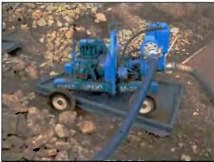
Poor work practice. The drip tray is undersized, constructed of too light a material, and accordingly overly flexible, easily damaged, and unlikely to retain oil residues.
