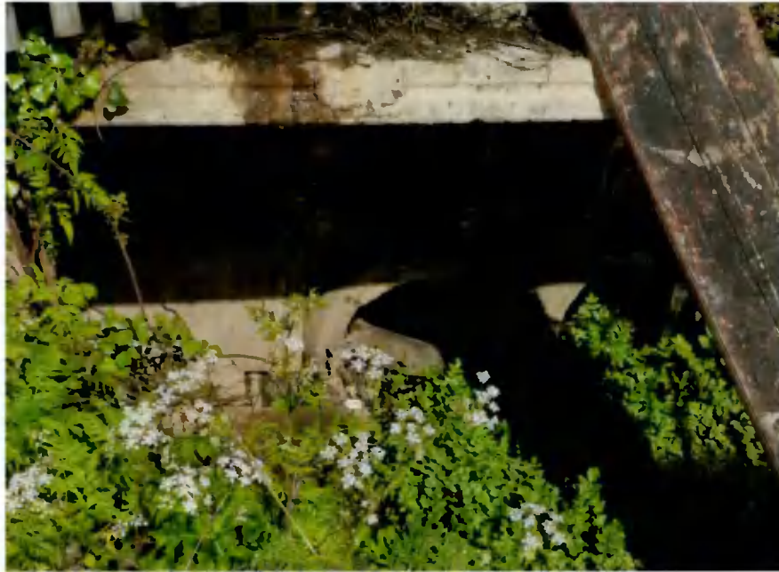
Fig 4 Picture Showing Culvert Below Neighbouring Site at The Downstream End of the Existing Stream
