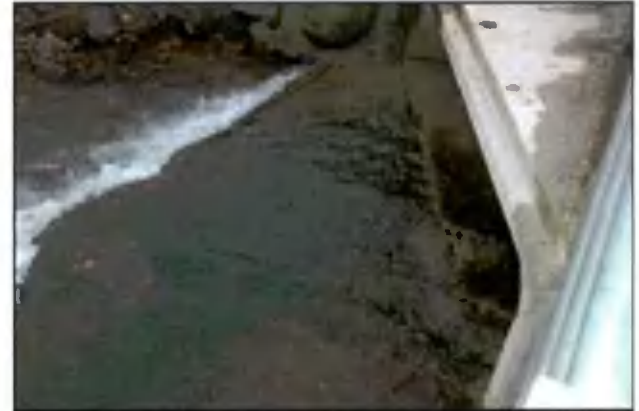
The smooth concrete finish is totally unsuitable for fish passage.
