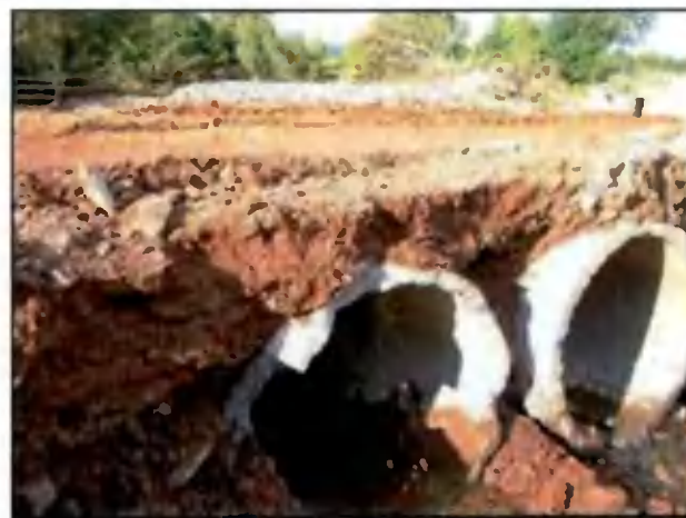
Temporary crossing structure. Impassable for aquatic life and emitting silt to waters as construction equipment traverses the crossing. Unacceptable practice.
