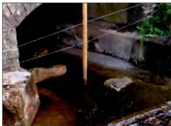
Large stone baffles held in position on concrete apron with stainless steel dowel rods drilled into both the apron and stones. (Poor placement of the livestock fencing as shown in the photograph has the potential to cause blockage by catching debris.)
