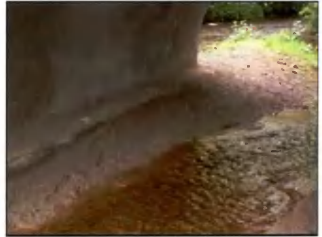
Gunite rebound on a stream bed where no precautions were taken to prevent its entry to waters. Rebound having a pH >11.5 would have entered the actively flowing stream with dire environmental consequences.
