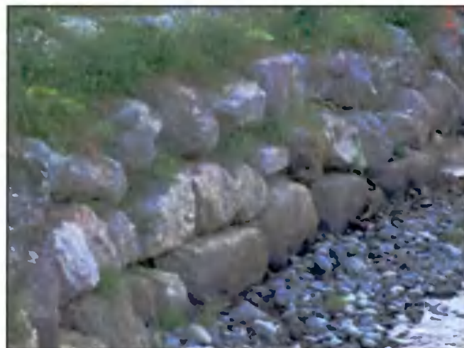
Revegetation of rock armour facilitated by the placing of locally sourced topsoil (to ensure no importation of non local grasses and shrubs) between each layer or course of boulders at installation time.
