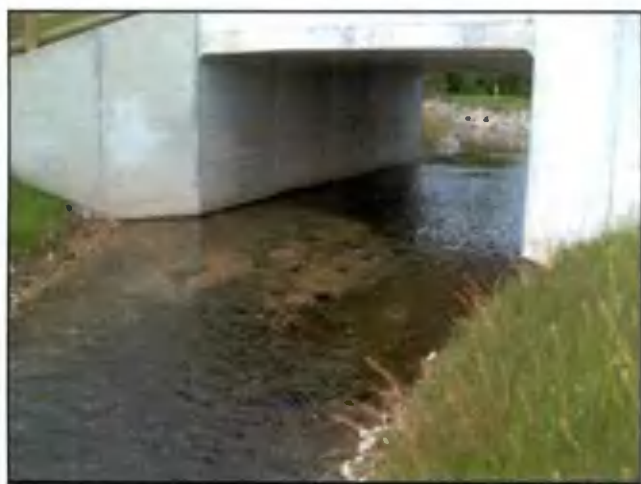
Excessively wide culverts can result in reduced current speed, ponding, and siltation of instream gravels.
