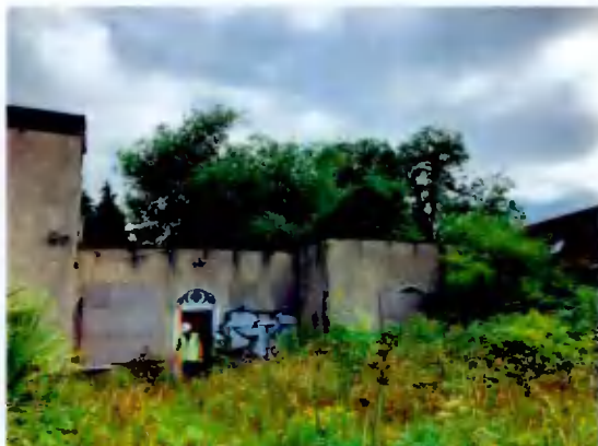
Part of front elevation showing stains at every parapet joint.
