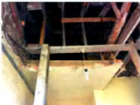
Interior missing/disturbed structural timbers.
