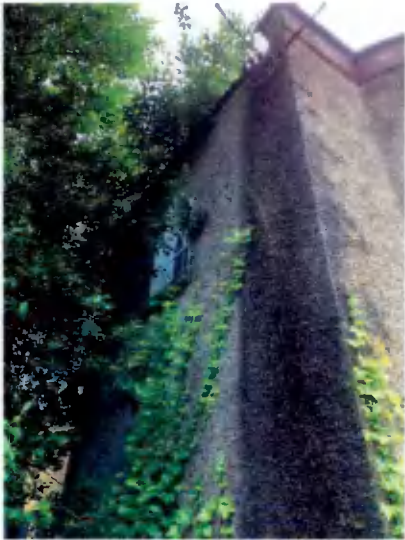
Rainwater staining at north east corner.
