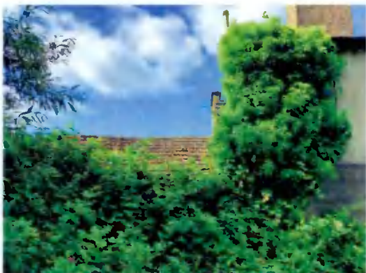
Bowed concrete tile roof.
