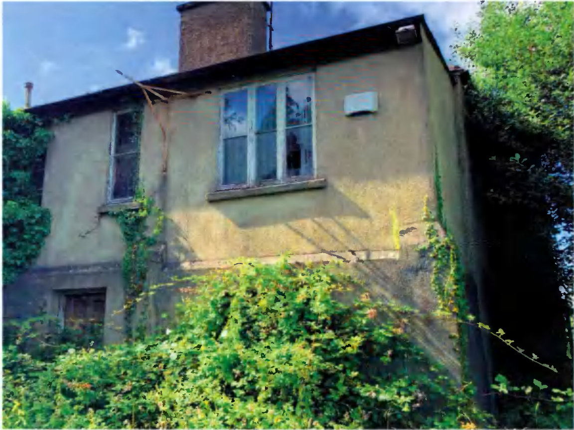
The rear elevation of the house - note projected ground floor wall face.
