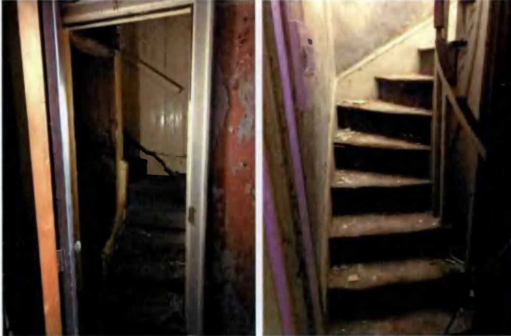
Existing stairs – note sagging tread.
