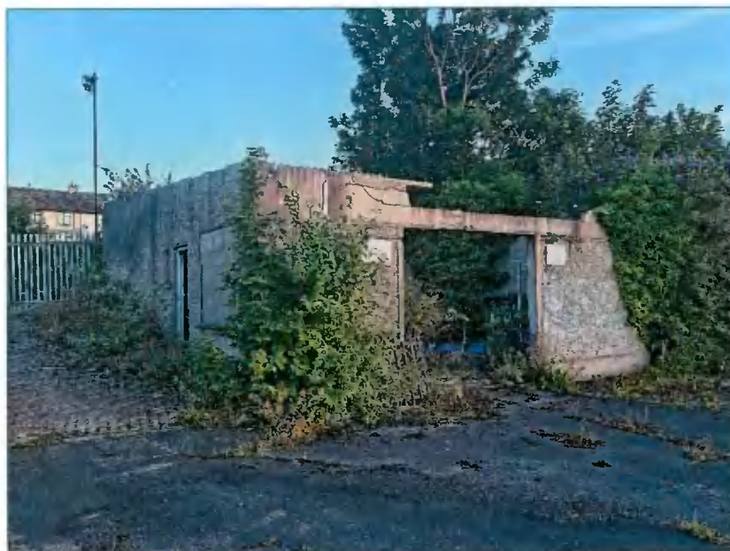
Plate 4. Derelict shed with no roof. Negligible bat roost potential.
