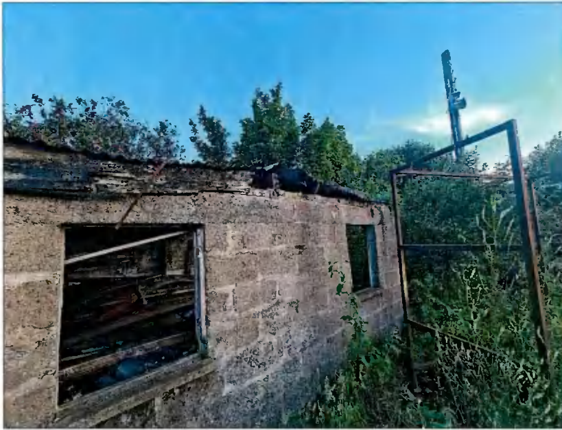
Plate 5. Second derelict shed on site with large gaps in the roof and rotting timberwork. Unsuitable for roosting bats.
