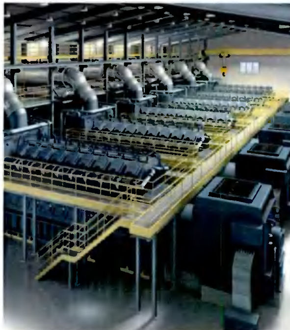
Figure 3-1 Typical Gas Engine Configuration
