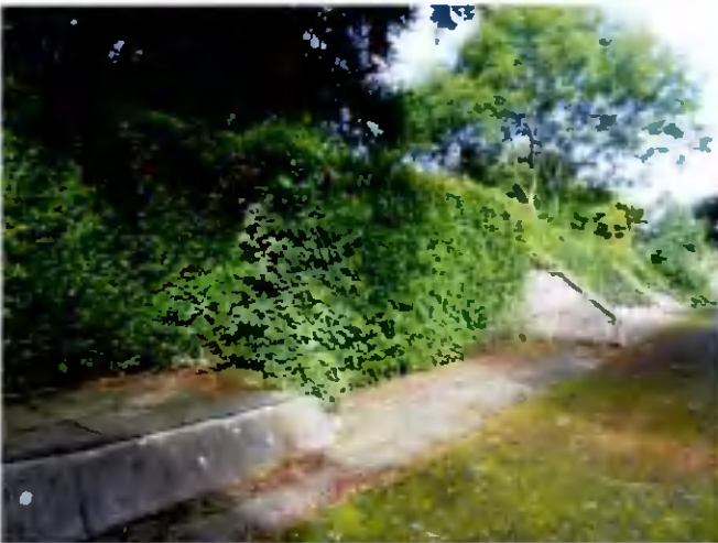
3.0m high – boundary wall to Coolamber. Buttresses to be reduced in depth and reinforced.
