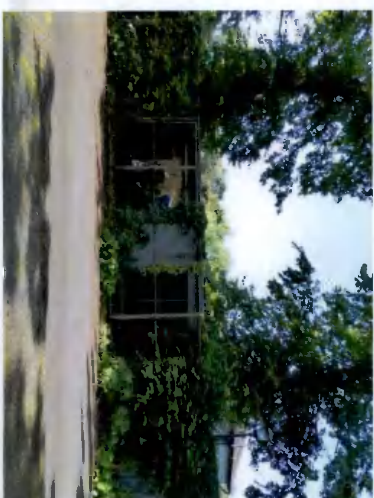
Fig 27. Garage/shed abutting flanking wall
