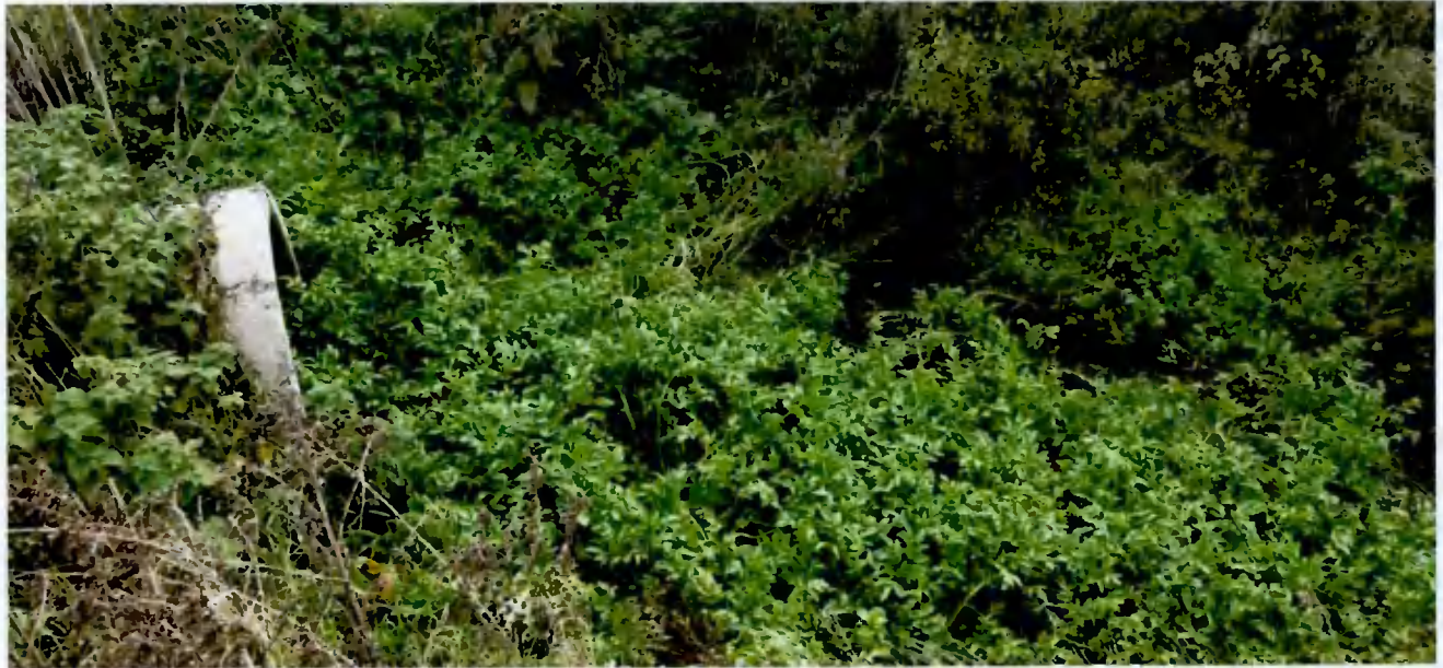
Figure 3-2: The drainage ditch running along the southern site boundary and joins with the unnamed River Griffeen tributary before entering the culverted system.
