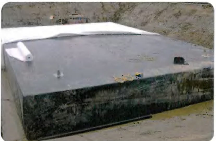
2mts deep tank with 3mts cover
