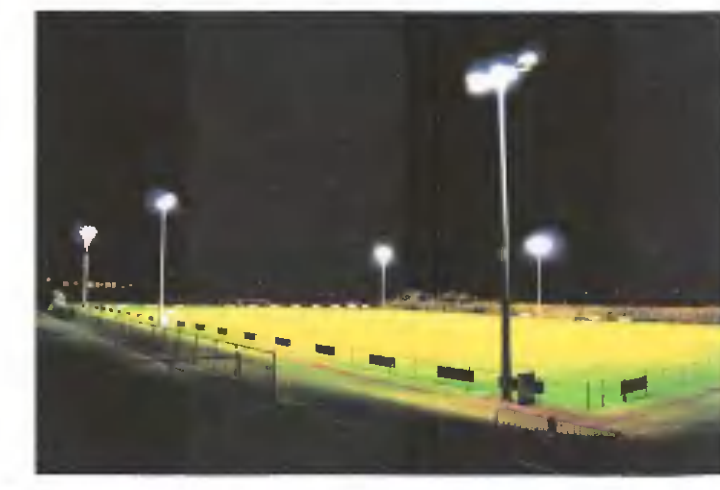
FLOOD LIGHT COLUMNS - Example Images only
