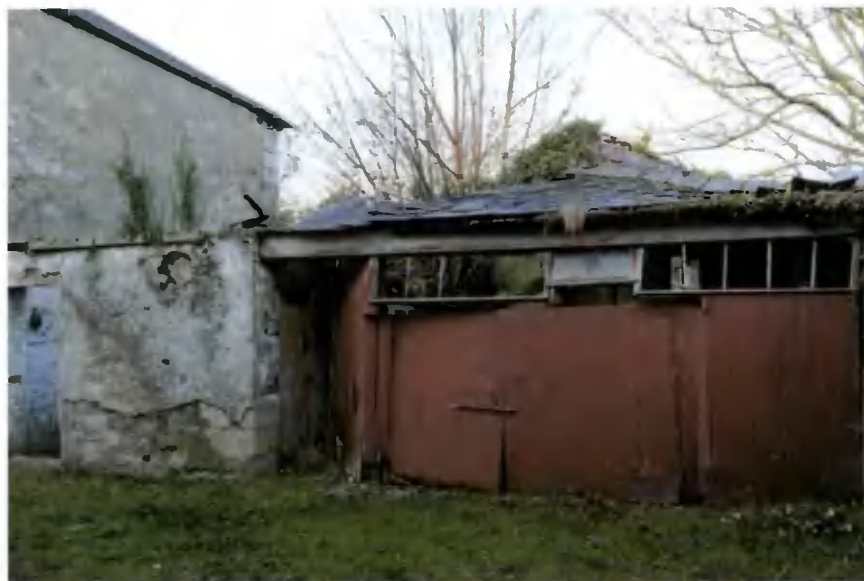
Plate 7: Rear of ruined building
