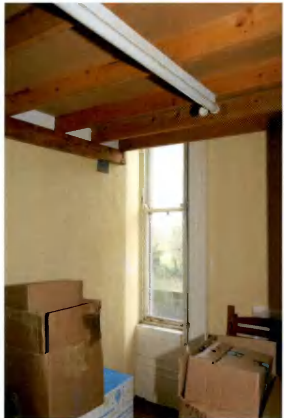
Plate 50: Window in room F-11
