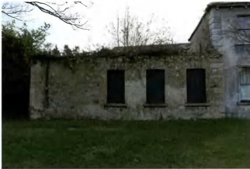
Plate 6: Front of ruined building
