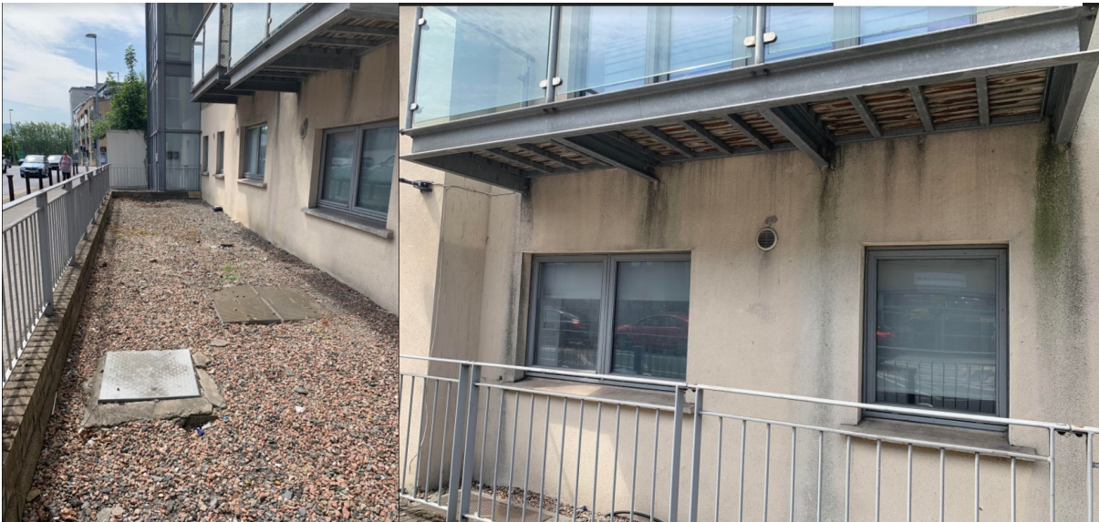
FIG. 2: POOR STREETScape INTEGRATION, NO PLANTING, POOR BUILDING MAINTENANCE, ETC.
