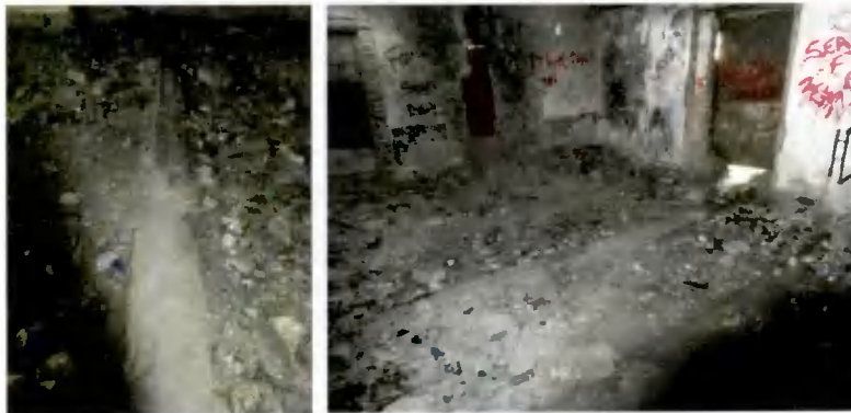
Figure 29: Remains of sleeper walls in Room G05
