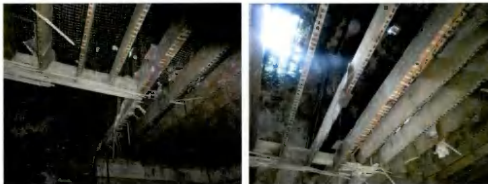
Figure 30: Stairs opening in first floor joists above Room G04 and above Room G01
