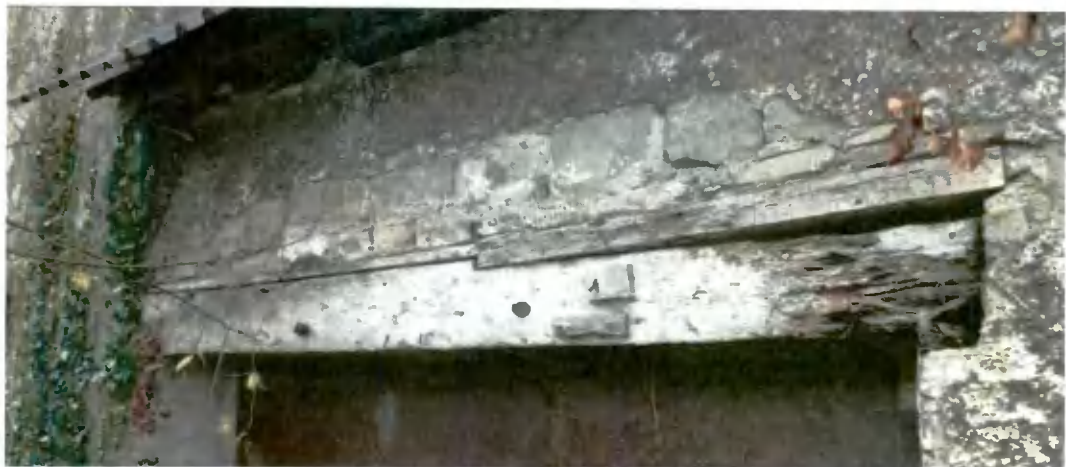
Figure 26: Decay of lintel over large window opening on south elevation
