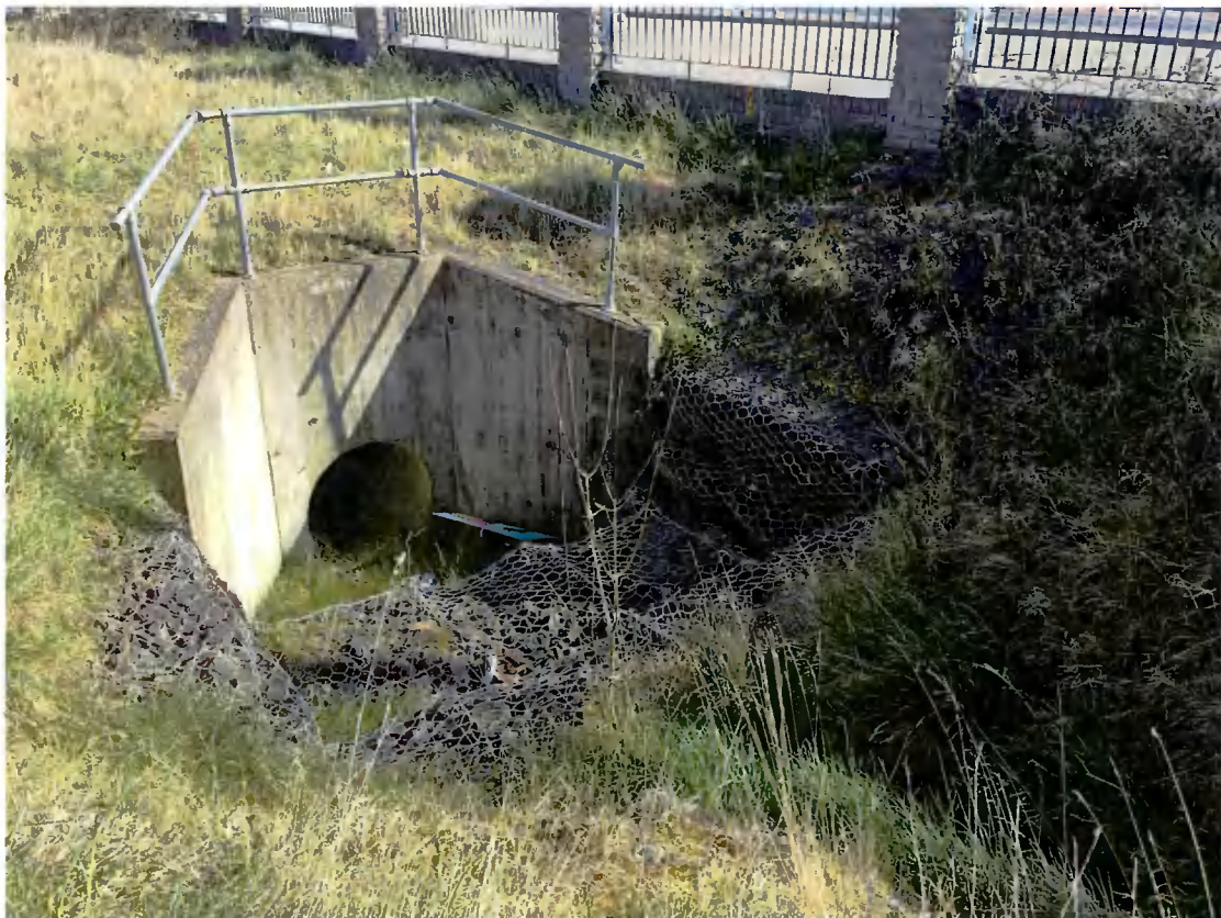
Photo 4. Culverted end of the more recently developed drainage ditch along the Outer Ring Rd. boundary (note: dry at this end in March after recent rain).
