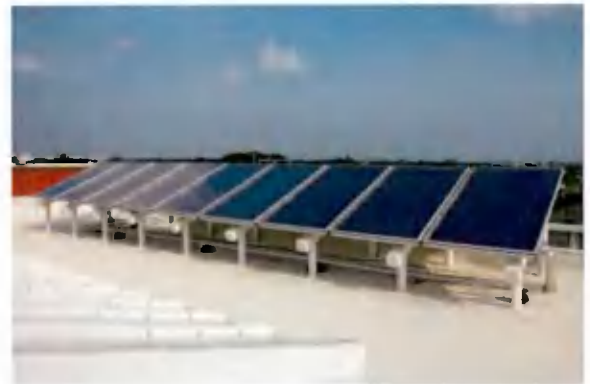
Glazed flat plate collectors
