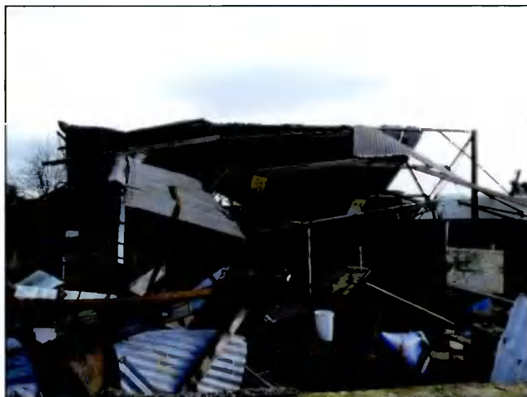
Figure 6.12 Collapsed farm shed in north of the Proposed Development site.
