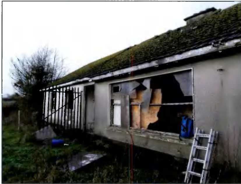
Figure 6.14 External view of derelict property in the northern side of the Proposed Development site.
